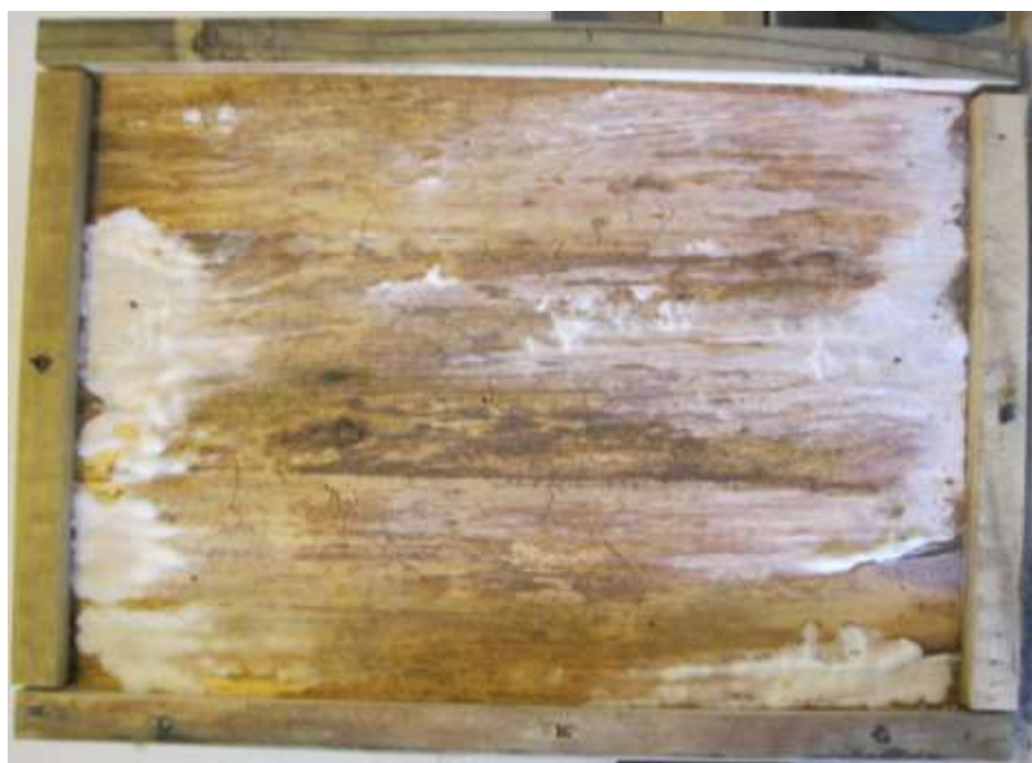
Figure 8 – The reverse side of untreated, assembly U1 after 28 weeks exposure. The fibre cement sheathing and building paper have been removed. Decay mycelium had spread across the whole of the surface. While the white mycelium appeared to be from the O. placenta feeder blocks there was dark, lace-like mycelium also on the surface suggesting infection by an outside decay fungus, possibly Coniophora puteana .
