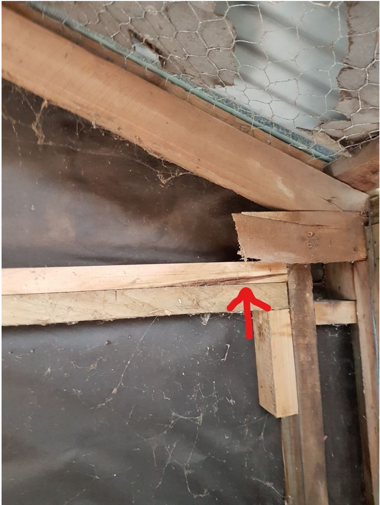
Macrocarpa sapwood showing bark encasement. No borer present.
