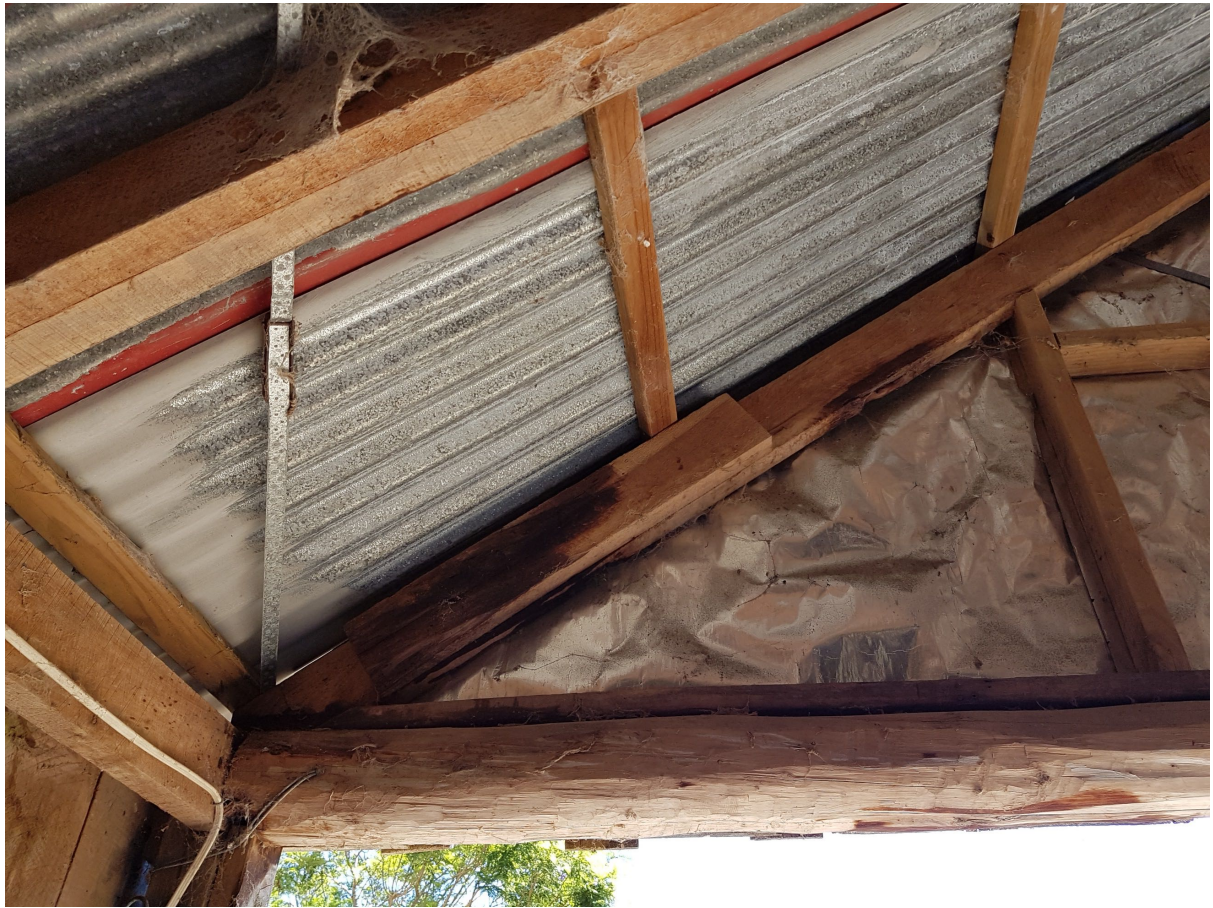
Macrocarpa beam from 50 year old tree, showing sapwood with no borer
