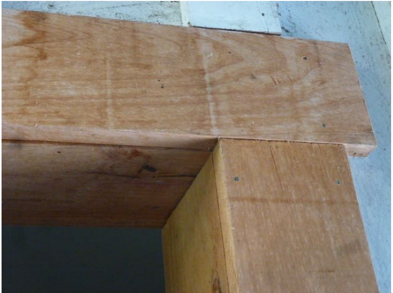
4" x 1" door surround of exterior washhouse (under partial cover, but note water stain as result of heavy wind during storms)
