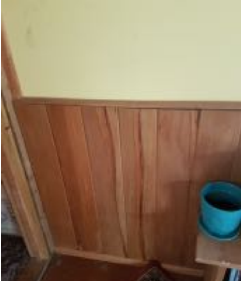
Rimu panelling showing borer
