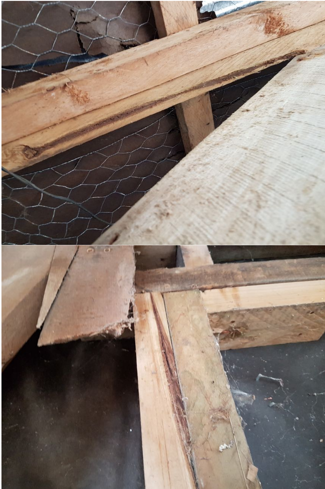
Macrocarpa sapwood showing bark encasement. No borer present.
